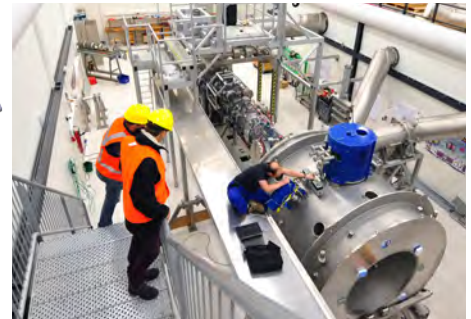
Superconducting magnet installed.
