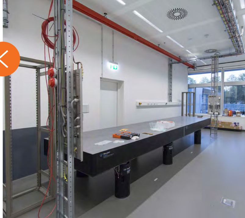
Installation of optical tables in a compartment of the Photonics-for-Energy-lab just after the reconstruction (September 2016)
